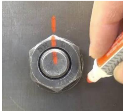
Figure 2: Example of bolt marking as a visual reference to verify loosening.
